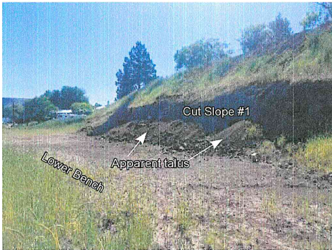
Photograph 9: Looking east at cut slope present at south side of lower bench of site.
