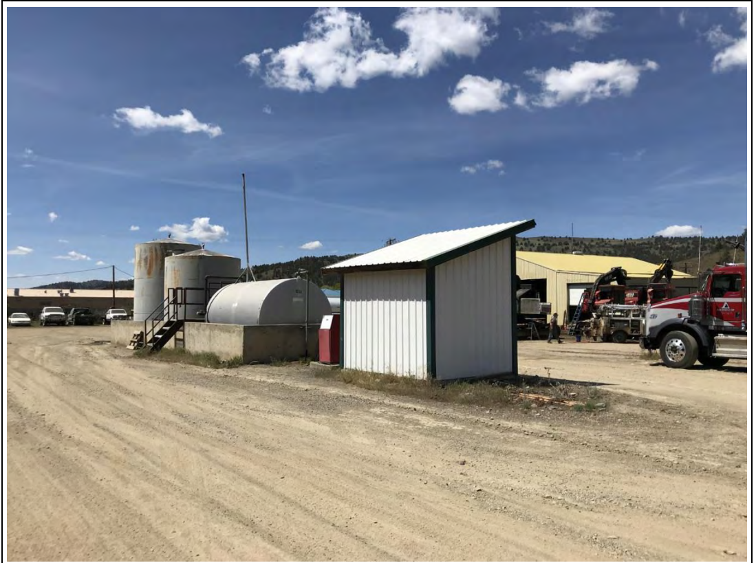
Above ground fueling station.
