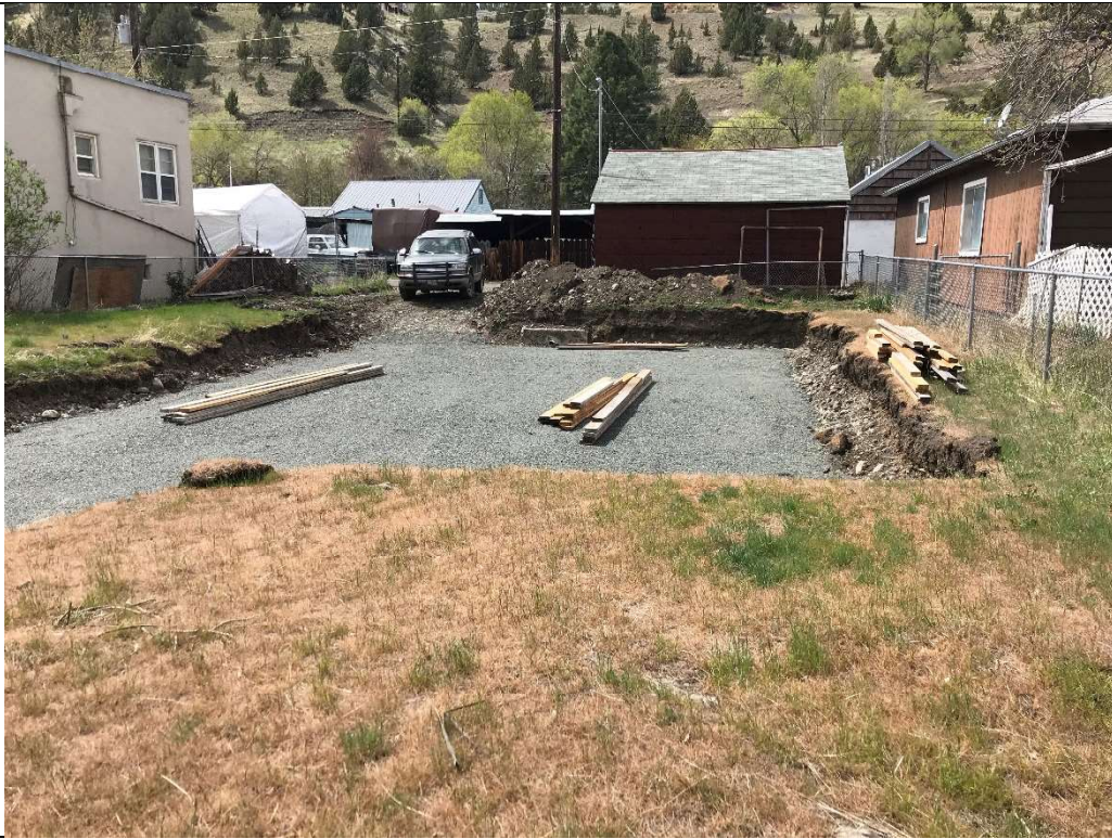
Photo 5. View of a house foundation excavation located approximately one-third mile north of the Project. The excavation shows a similar profile with finer-grained materials at the surface and coarser-grained materials underneath.
