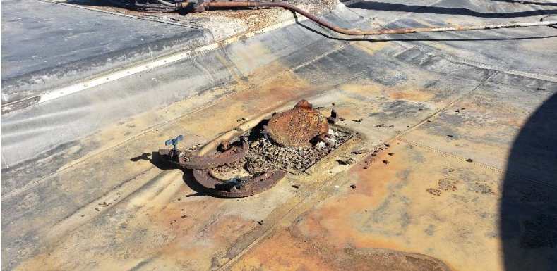
Photo 4 - Primary Digester roof – penetration failure – passive venting
