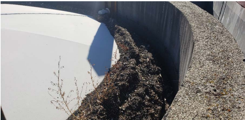
Photo 5 - Secondary Digester roof – failed floating lid
