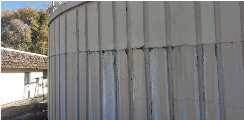
Photo 1 – Primary Clarifier – concrete cracking/weeping
