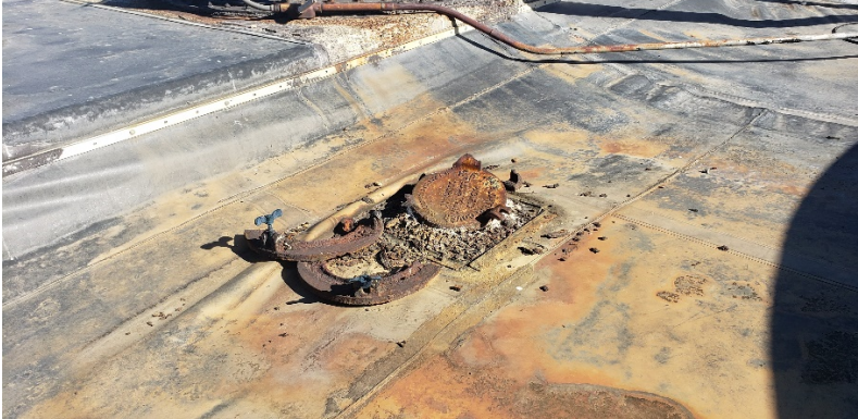
Photo 4 - Primary Digester roof – penetration failure – passive venting
