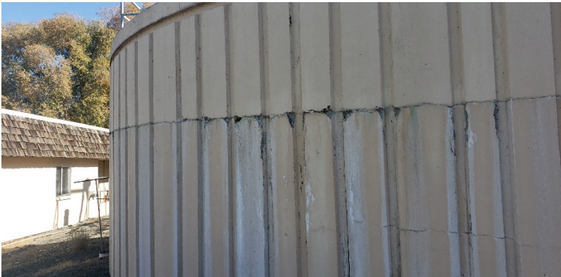
Photo 1 – Primary Clarifier – concrete cracking/weeping
