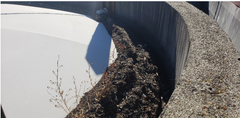
Photo 5 - Secondary Digester roof – failed floating lid
