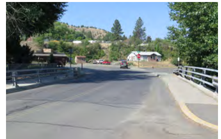
3rd Ave bridge over Canyon Creek provides sidewalks on both sides but lacks bicycle facilities.
