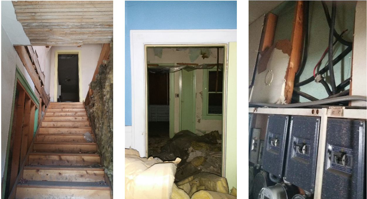
Figure 2. Interior stairwell (left); exterior walls and windows on interior of structure (middle); exposed interior electrical paneling and power meters (right)
