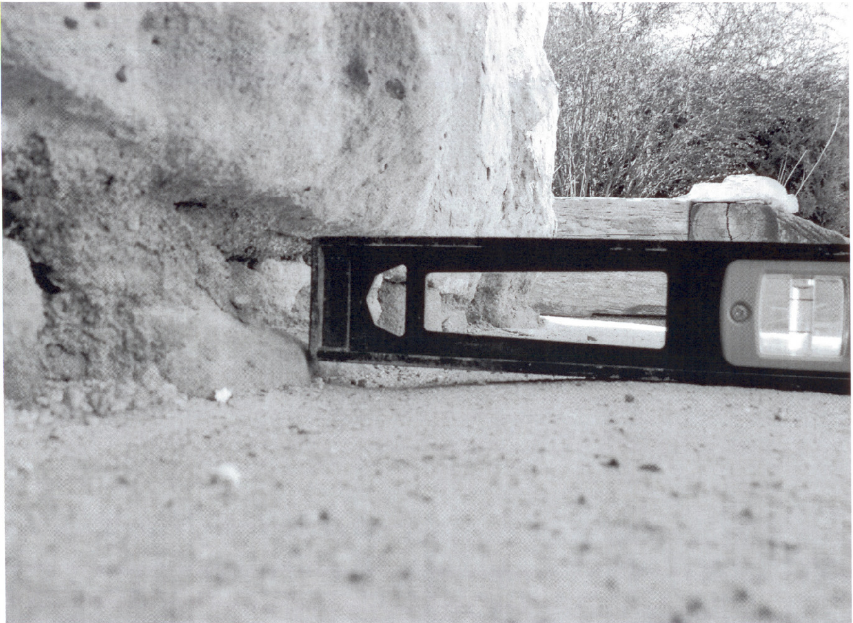
Photo 2. "rollover" of concrete near building trapping water; erosion of building foundation
