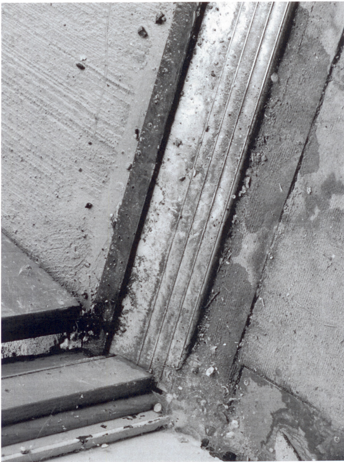
Photo 9. Water penetration of building from sidewalk higher than floor level and sloping to building
