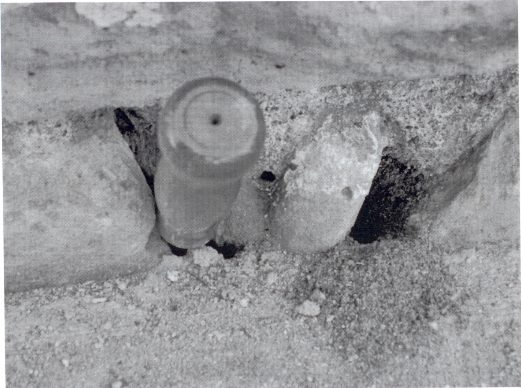
Photo 8. Water penetration of foundation from sidewalk; erosion of lime mortar; no expansion joint; hard concrete adhered to soft stone
