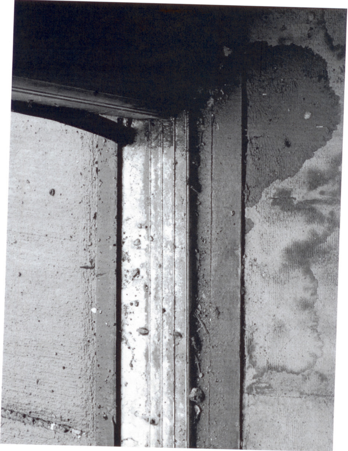
Photo 10. Water penetration to building
